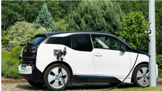
Fig. 8. Charger in the lighting pole [8]
